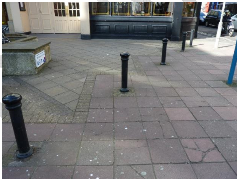
Bartholomew Square: incoherent street surfaces poorly maintained
